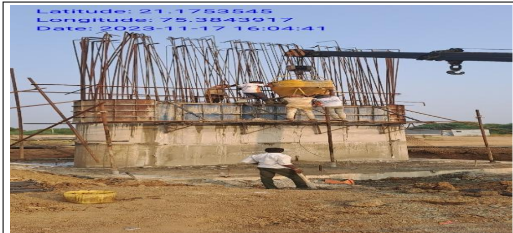
Photograph-3-Incomplete bridgework over Tapi river in Bhokar village
